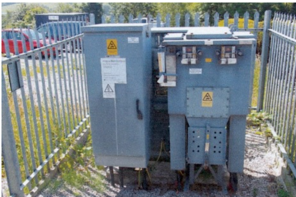
Fig.4. Hague Bar Outdoor substation (338852). It replaced a kiosk which was adjacent.
