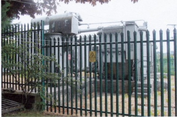
Fig.1. Gowhole 33kV substation 33kV 301671, on Lady Pit Road SK011838. This will not be the original equipment from 1930.
